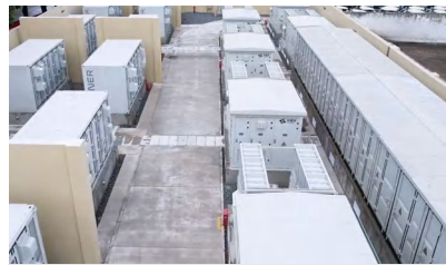
► C&I | Electromechanical Industry Jiangsu | 18MW/54MWh
