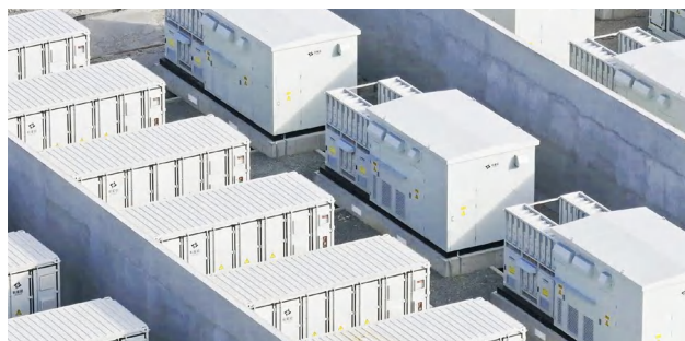
📍 China 🏗️ Grid-Energy Storage Project 📊 109.5MW/219MWh
