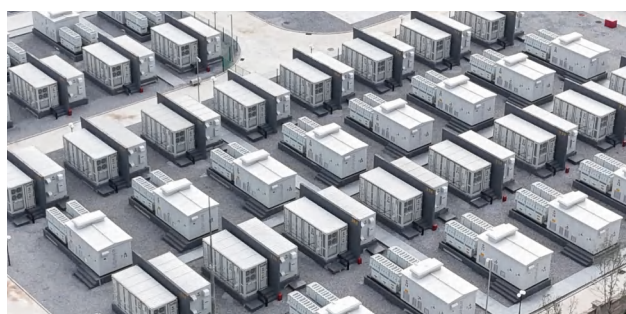
📍 China 🏗️ Grid-Energy Storage Project 📊 100MW/200MWh
