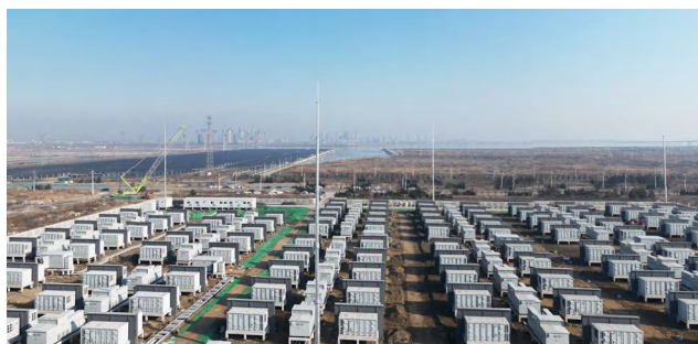
📍 China 🏗️ Grid-Energy Storage Project 📊 300MW/1200MWh
