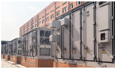
► C&I | Chemical Industry Zhejiang | 41MW/82MWh
