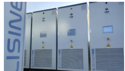
► PV+ESS All-in-One Smart Microgrid Project Chongqing | 2.3 MWp PV + 6.96 MWh ESS
