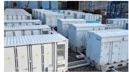
► C&I | Steel & Metal Jiangsu | 40MW/120MWh
